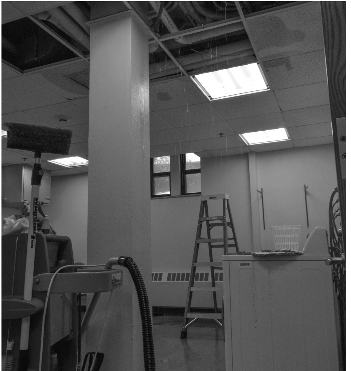
As the snow began melting, water started pouring from the ceiling in the Uhler laundry room.
